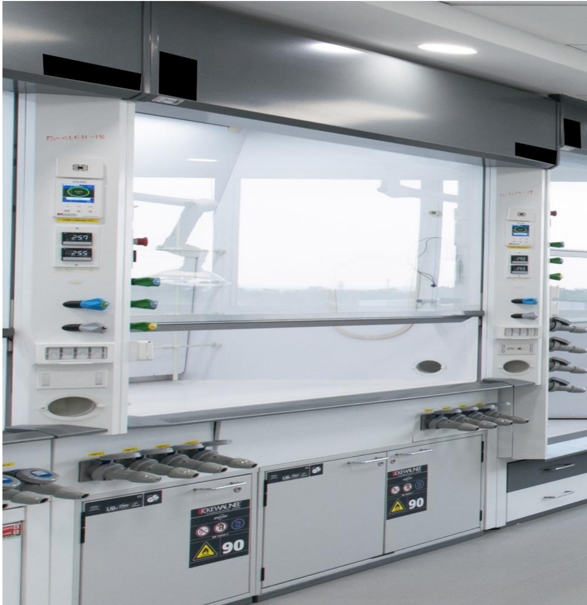
FIG: 15 Fume Hood with FM approved Solvent storage cabinet
